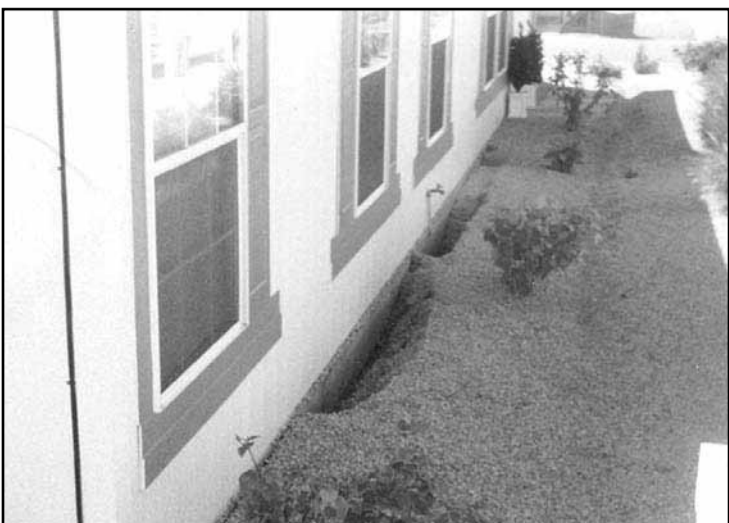
Sinkholes, as pictured above, plague homes in the Desert Harbor community.
